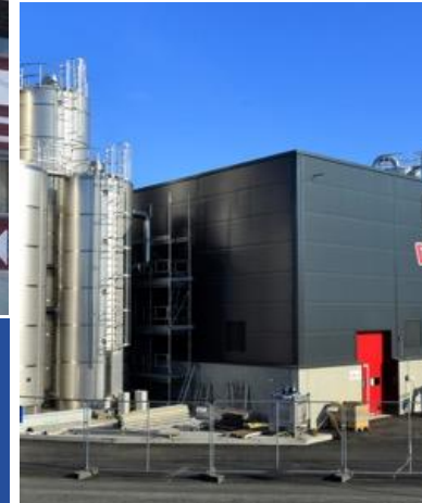
Industrial Applications & District Heating
