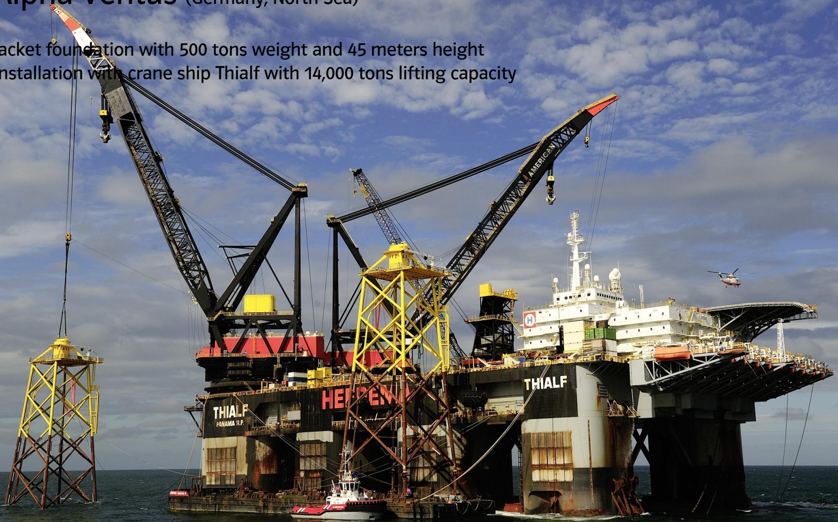
Jacket foundation (500 tons)
